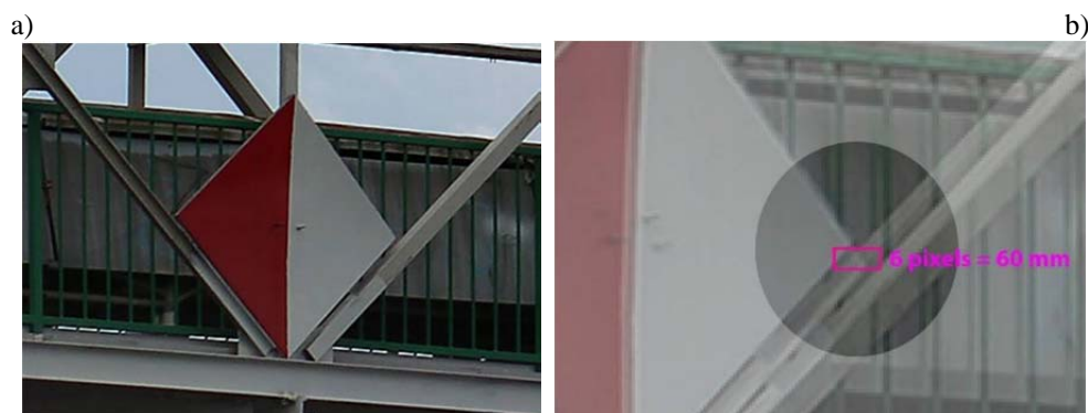
Fig. 9: The analysed detail in 1/2 of the bridge span: a) without load, b) overlap of two sequences of photographs (without and with load) showing the scale of the bridge displacements.
