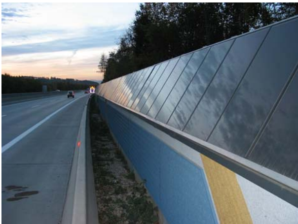
Fig. 5: the new wall with integrated photovoltaics
