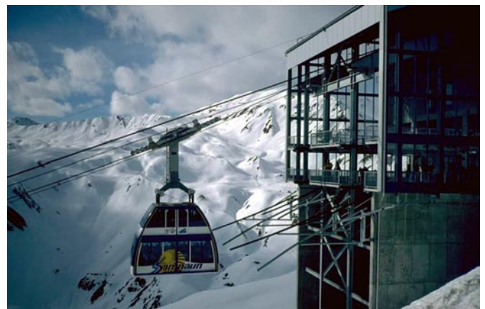
Construction of a new ski lift in France: A generalized development can be observed throughout the Alpine space which highly depends on globally determined location qualities.
