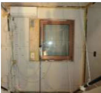
Inside view of wall with integrated micro heat pump (Project iNSPiRe)
