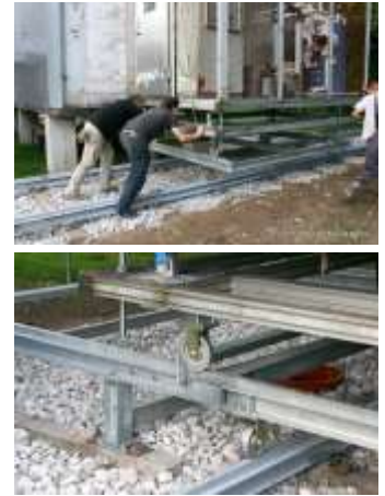
Rail system for placement of the movable Cold-Box
