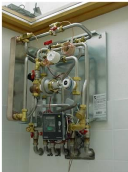
Heat delivery station for flat
